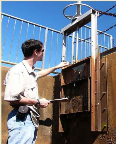
WSSI engineer inspecting the condition of a dam principal spillway on North Fork - Haymarket, VA
